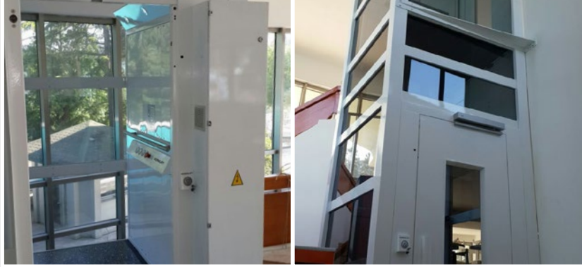
Vertical Wellless Lift /// İstanbul
